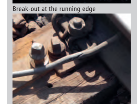
Loose rail fastening
